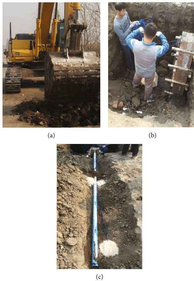
FIGURE 18: Monitoring tube embedding process underneath a section of a test roadway: (a) trenching; (b) concrete column pouring for anchoring cantilevers; (c) laying of a monitoring tube.
