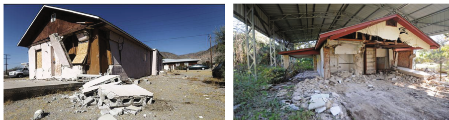
FIGURE 2: Seismic damage to an assembled concrete frame structure during an earthquake.
