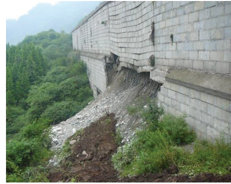
FIGURE 1: Failure of reinforced retaining wall in Wenchuan earthquake.
