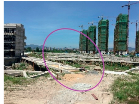
FIGURE 4: The Evergrande foundation pit located near the south side of the standard section of the foundation pit in the subway station.
