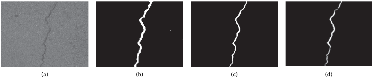
FIGURE 15: Longitudinal crack segmentation model results: (a) original image; (b) before improvement; (c) improved result; (d) ground truth.
