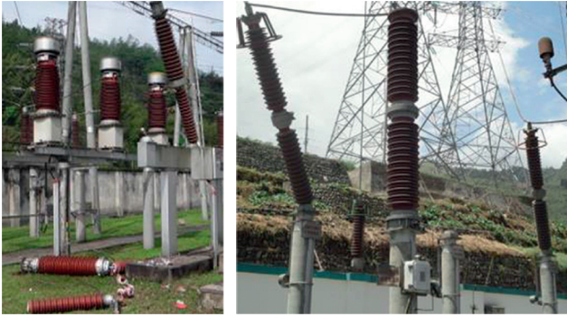
FIGURE 1: Seismic damage to pillar-type porcelain insulators.
