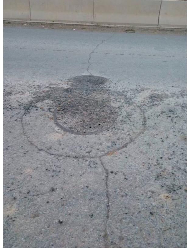
FIGURE 1: Crack of asphalt pavement structure.
