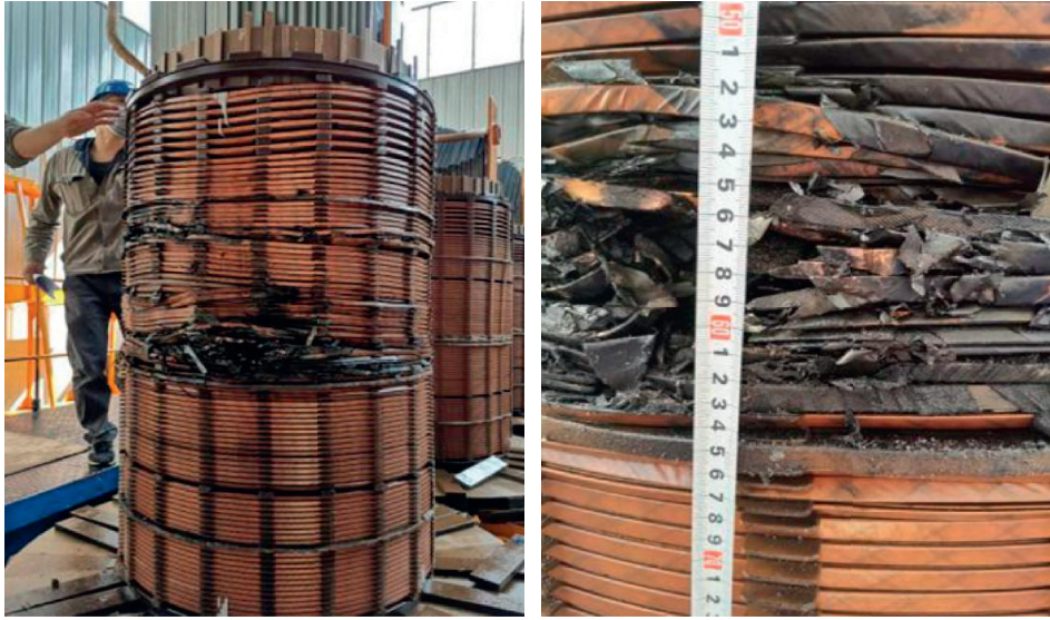
FIGURE 9: Burning loss between turns of A phase low voltage coil.
