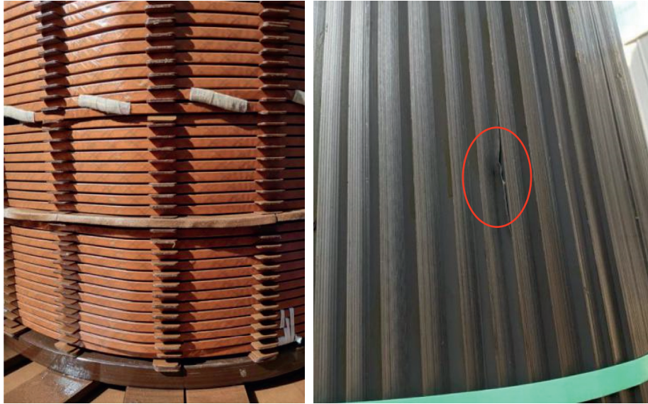
FIGURE 12: C phase low voltage coil and silicon steel sheet deformation.
