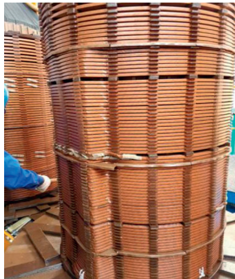
FIGURE 11: B phase low voltage coil bulge.
