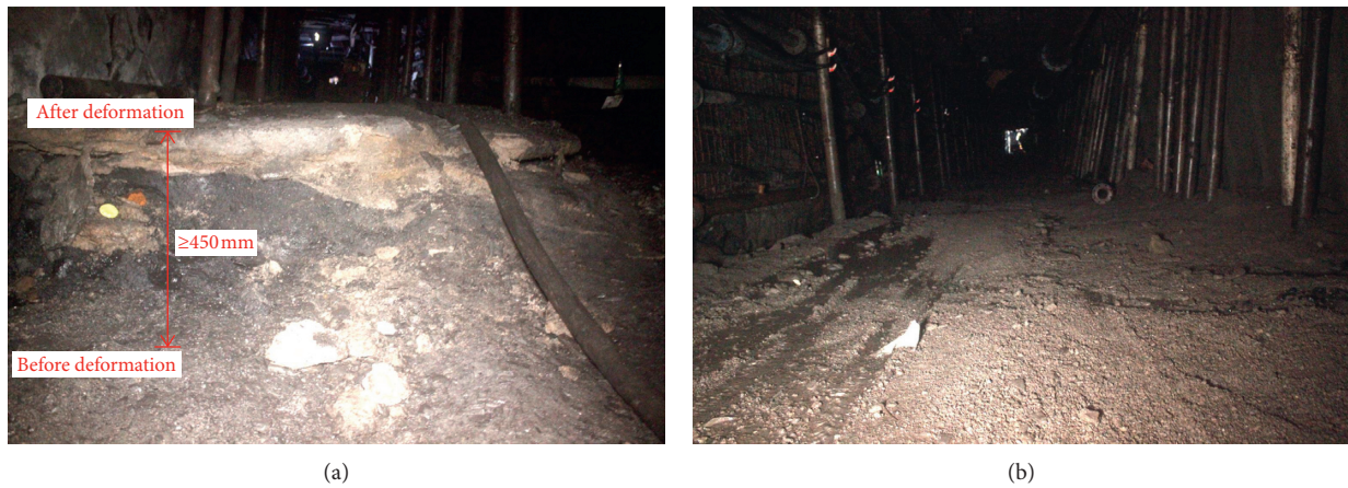
FIGURE 20: The control effect on floor heave. (a) Before control. (b) After control.
