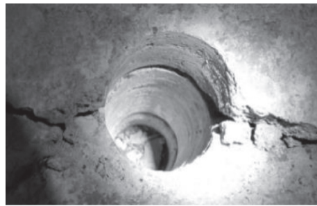
FIGURE 7: Crack in the fill layer.
