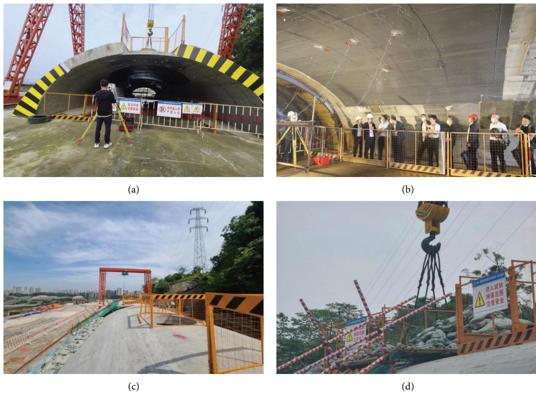
FIGURE 12: Construction safety control. (a) Tunnel model entrance isolation. (b) Tunnel model internal isolation. (c) The tunnel model was fully enclosed and isolated. (d) Warning signs around the vault test block.
