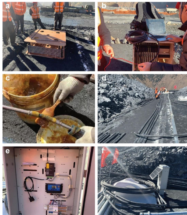
FIGURE 3: Photographs of embedding the SAA at the construction site. (a) Transport the packaged SAA to the construction site. (b) On-site SAA inspection. (c) Apply butter to the SAA and place it in the PE pipe. (d) Burying the SAA in the trench. (e) Solar power generation system. (f) Connection between generation system and SAA.
