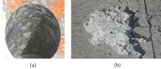
FIGURE 4: Concrete deterioration: (a) bridge deck delamination in a drilled hole and (b) bridge deck degradation due to alkali-silica reaction [49].
