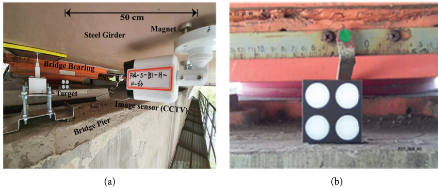
FIGURE 6: Displacement monitoring system: [66] (a) configuration of the measurement system and (b) target installed on bearing support.
