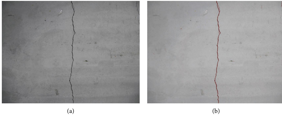
FIGURE 14: The constructed method applied to full-scale bridge crack image detection. (a) Original image. (b) Crack segmentation result.
