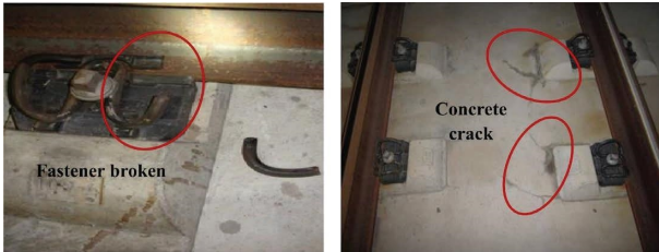
FIGURE 2: Ballastless track surface defects: (a) fastener broken [3]; (b) concrete crack.
