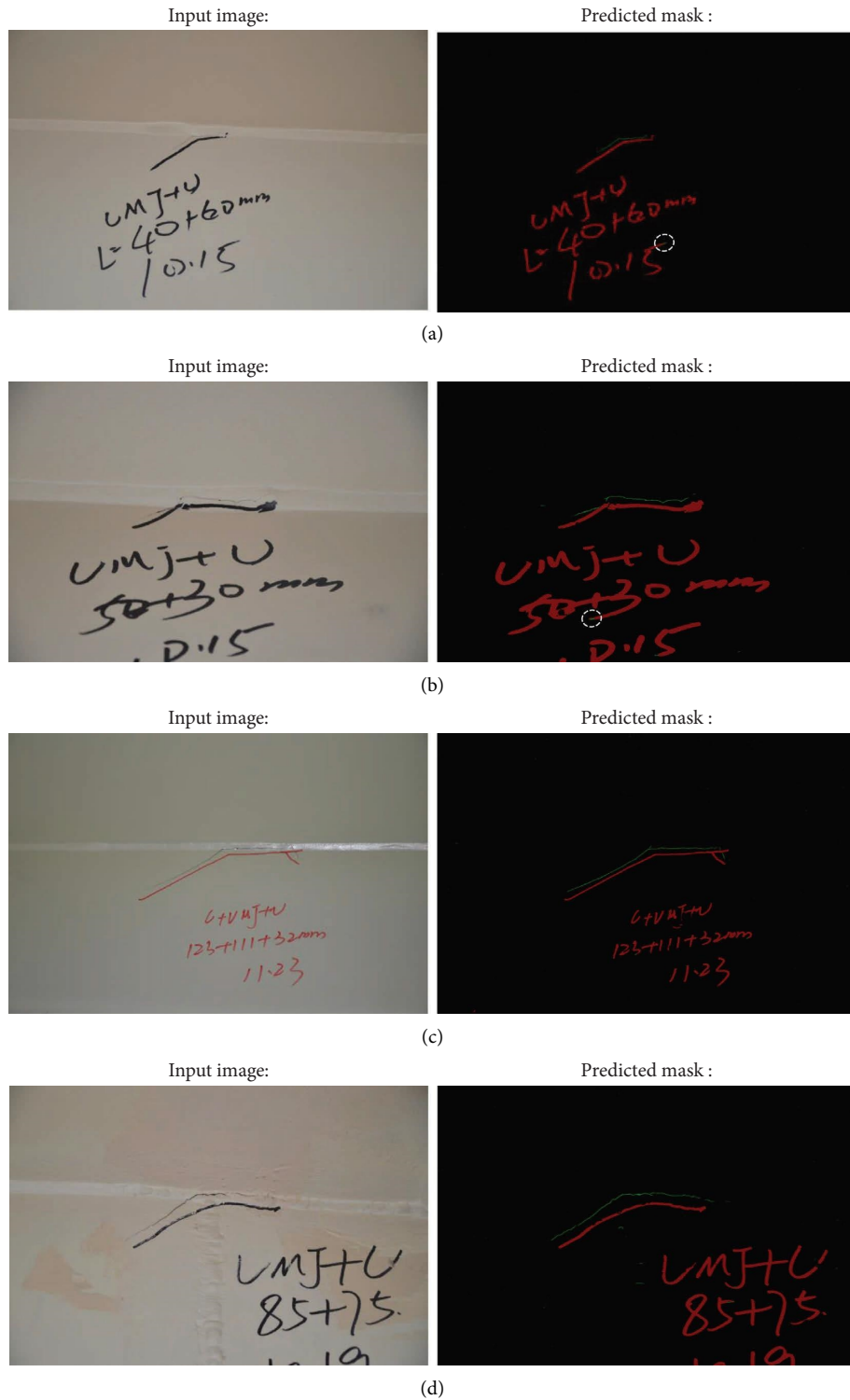
FIGURE 11: Original-image segmentation results for idea inspection conditions: (a) subtle crack, (b) fine crack, (c) medium crack, and (d) coarse crack.
