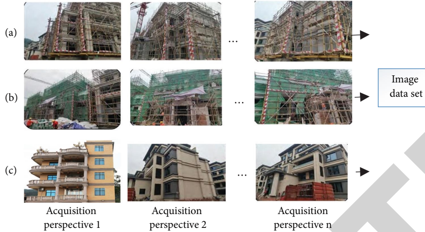
FIGURE 3: Real-time image data of the construction site from various angles: (a) construction of scaffolding on an exterior wall; (b) construction of protective net on an exterior wall; (c) construction of paint on the exterior wall.
