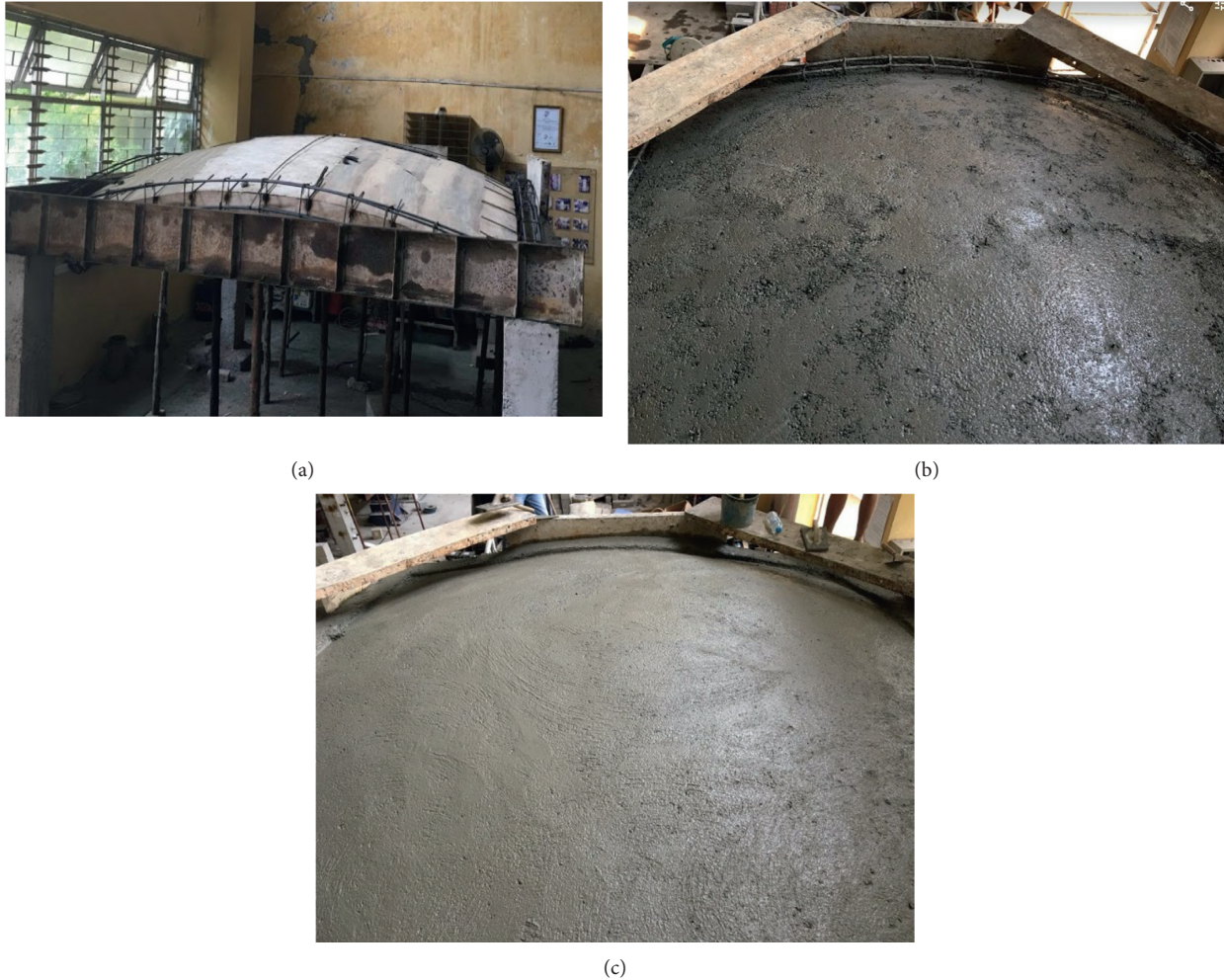
FIGURE 2: Making the formwork and pouring concrete layers: (a) make the formwork, (b) the first layer of steel fibres concrete was poured, and (c) the normal concrete layer is poured last.
