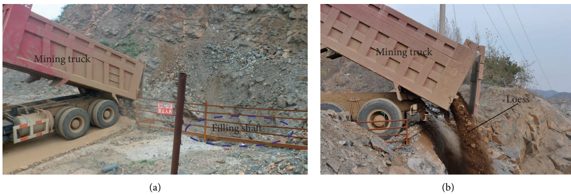
FIGURE 4: The filling process by mining truck. (a) Waste rock filling. (b) Loess filling.
