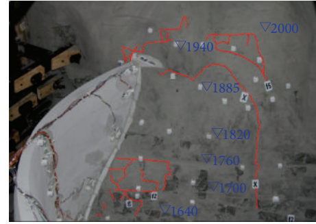
FIGURE 11: Failure patterns of the left abutment ( K_2 = 7.6 ). Note: the red lines show the cracks in the model.
