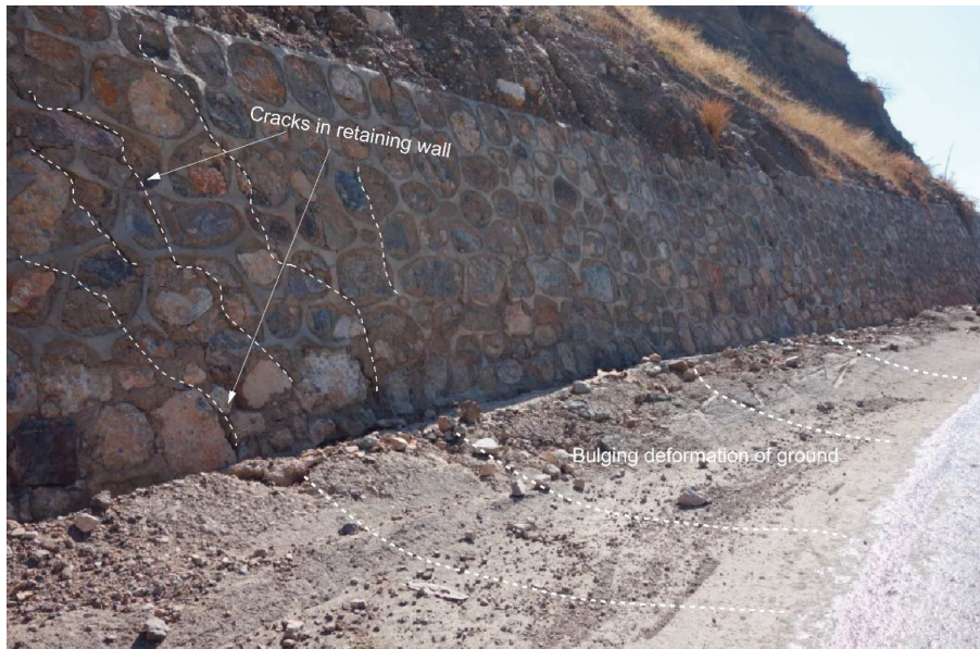
FIGURE 10: Cracks in the retaining wall and bulging deformation of the road.
