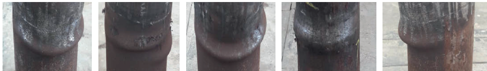
FIGURE 7: Local buckling of the steel tube.
