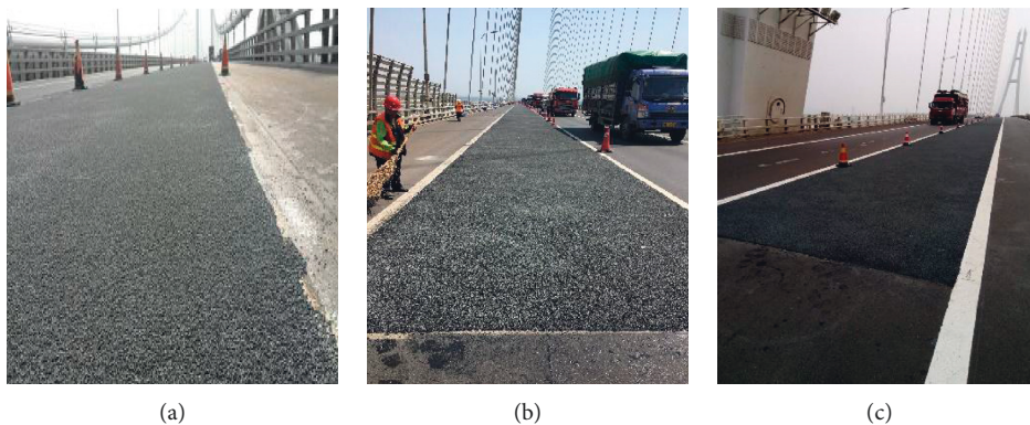
FIGURE 21: Effects of construction. (a) Zhenjiang–Yangzhou Yangtze River Bridge (2014). (b) The third Nanjing Yangtze River Bridge. (c) Suzhou–Nantong Bridge.
