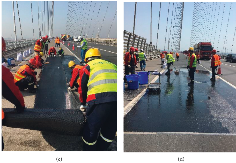
FIGURE 20: Construction technology of the thin overlay of fiber-reinforced resin on the Suzhou–Nantong Bridge.
