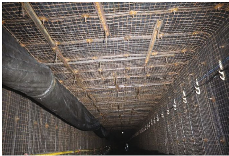
FIGURE 18: Roadway surrounding rock control effect.
