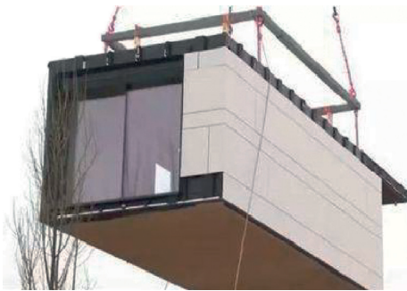
FIGURE 2: Hoisting and installation of a modular prefabricated building prototype (source: authors' own data).
