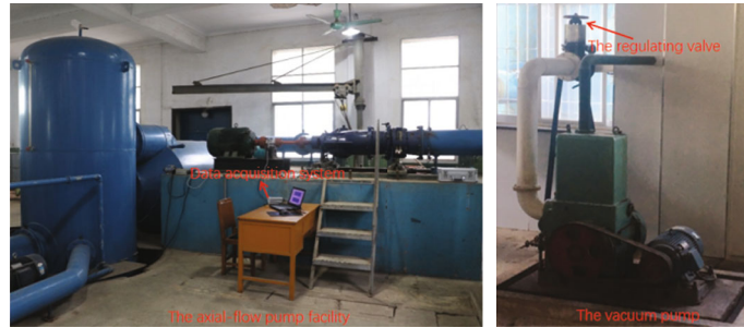
FIGURE 1: Experimental pump station installed in the Wuhan University.
