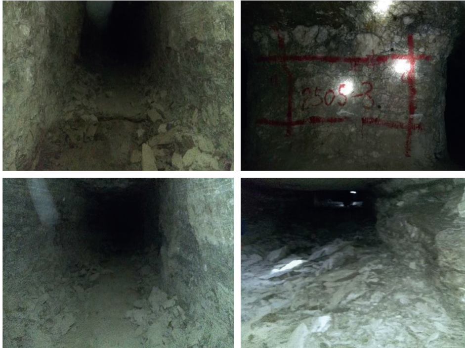
FIGURE 6: Weathering damage of gypsum mine pillars.
