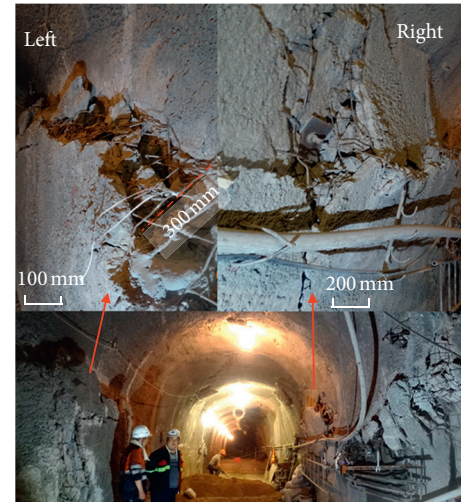
FIGURE 1: Large area of extrusion cracking on the sidewall of the deep tunnel.
