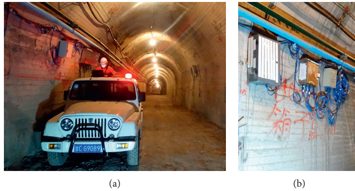
FIGURE 14: Data connection of field equipment. (a) Data link field operation and (b) data acquisition module.
