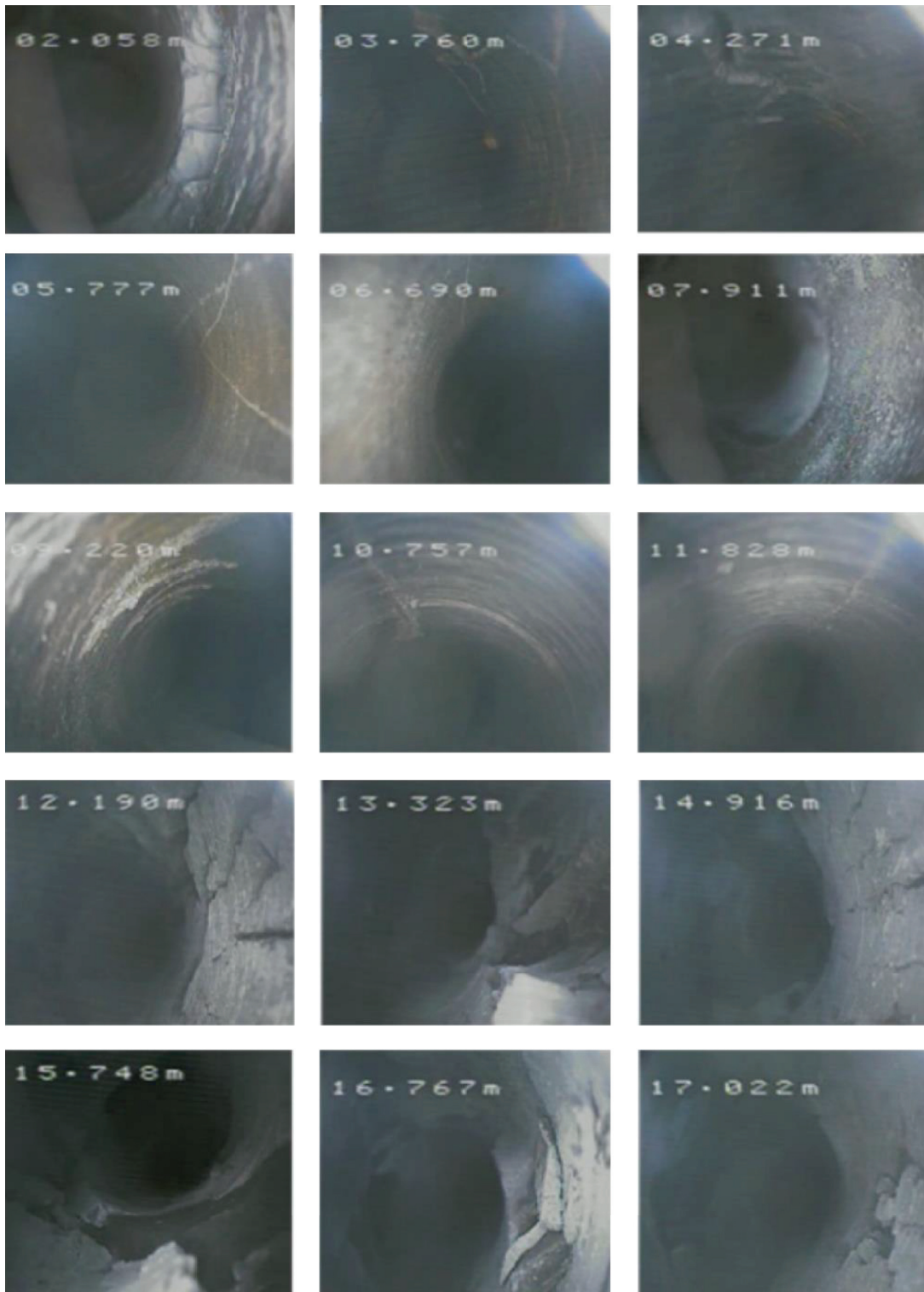
FIGURE 25: The inner surface of the surrounding rock in the blast borehole.
