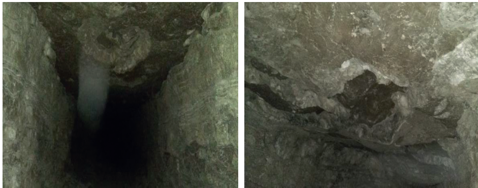
FIGURE 4: Weathering damage of a gypsum mine room.
