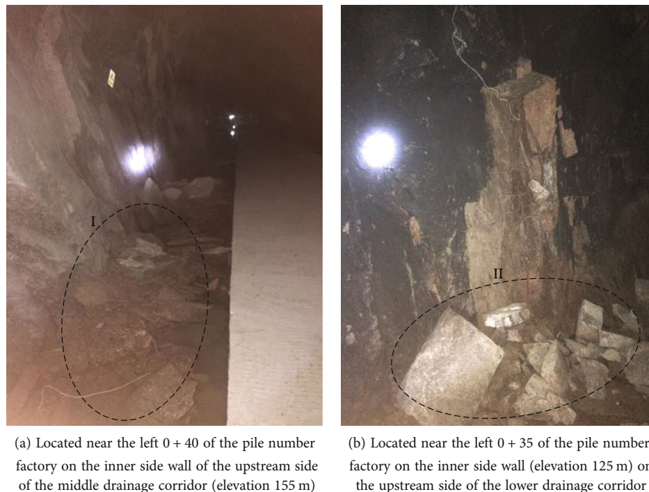
FIGURE 11: Collapses of rock mass in microseismic accumulation area.
