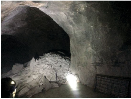
FIGURE 2: Rockburst at the intersection between lower drainage corridor and tailrace branch tunnel no. 1.
