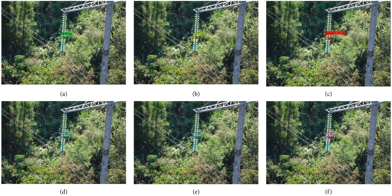
FIGURE 7: Defective suspended glass insulator detection.
