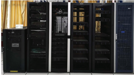
FIGURE 4: Microseismic monitoring center.
