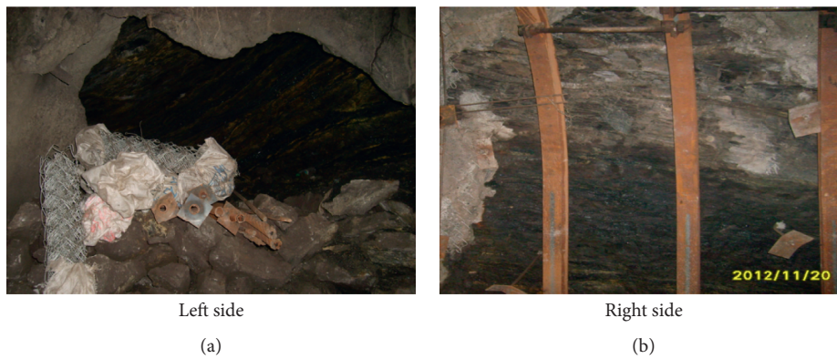
FIGURE 5: The damage of the surrounding rock. (a) Left side. (b) Right side.
