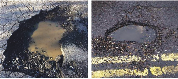
FIGURE 1: Road image having potholes [2].
