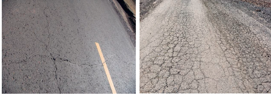
FIGURE 1: Crack distresses in Qinghai-Tibet Highway.
