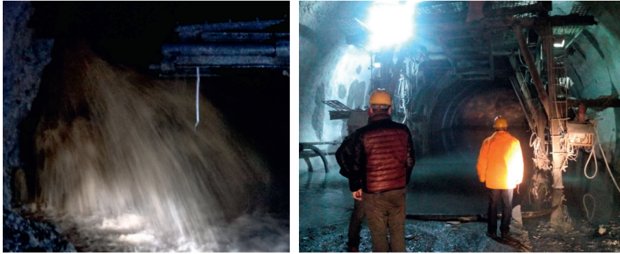
FIGURE 12: Photos of water gushing from actual excavation to K42 + 530.
