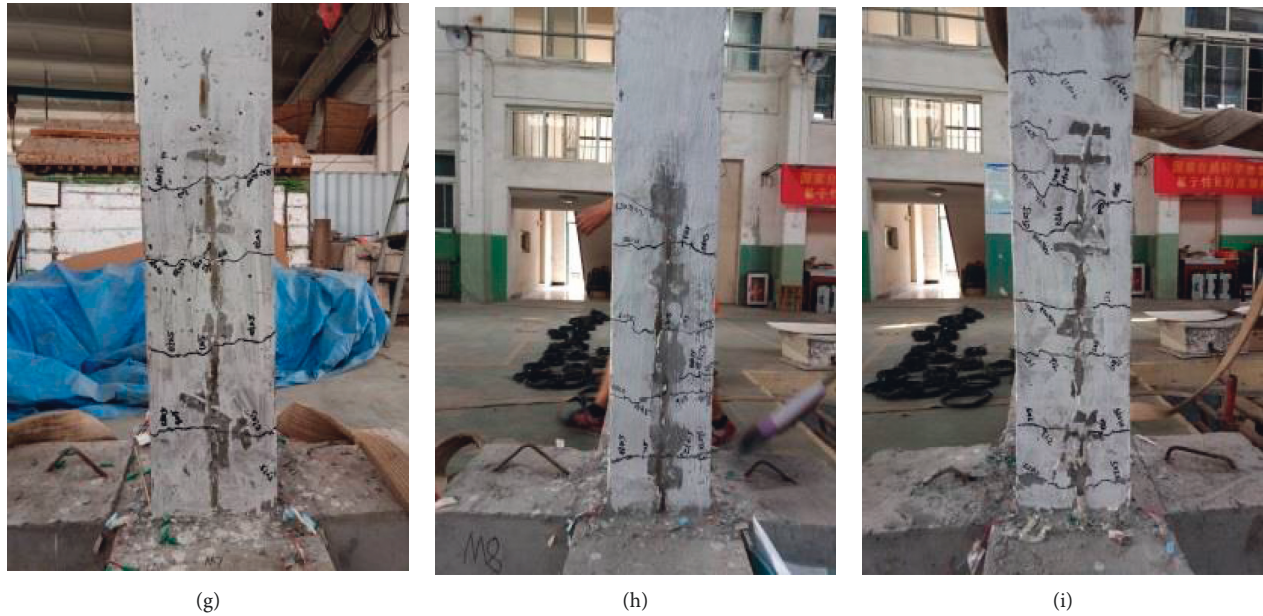
FIGURE 6: Distribution of postearthquake cracks of each pier: (a) M1; (b) M2; (c) M3; (d) M4; (e) M5; (f) M6; (g) M7; (h) M8; (i) M9.
