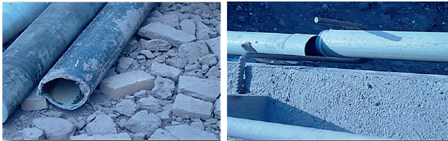
FIGURE 4: Damage occurred from Manjil earthquake.
