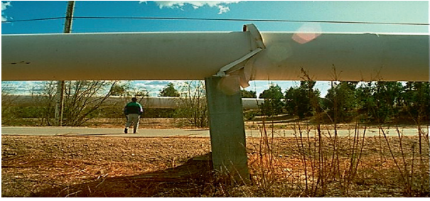
FIGURE 10: Demolition of pipes' support due to soil liquefaction in the Northridge earthquake (1994).
