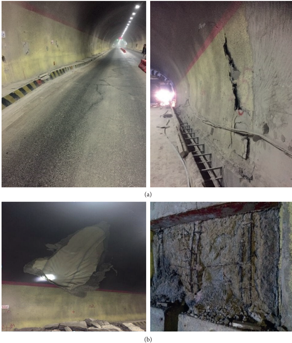
FIGURE 6: Photos of different damage degrees for Dugongling tunnel. (a) Initial damage of tunnel lining. (b) Further damage of tunnel lining.
