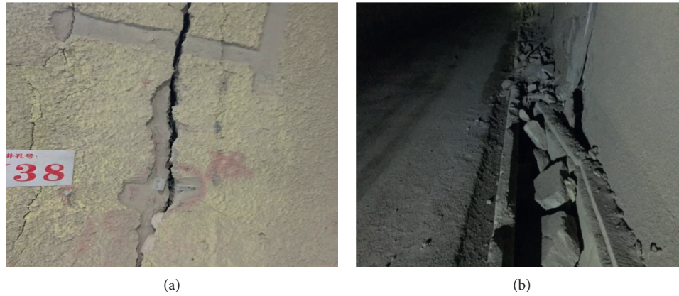
FIGURE 10: Tunnel diseases in November 2013. (a) Lining cracking. (b) Movement of cable duct.
