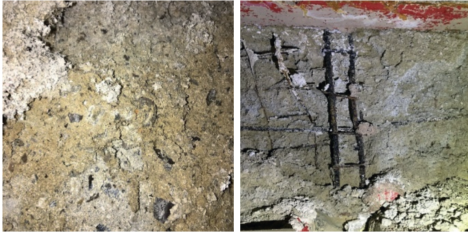
FIGURE 5: Corrosion of tunnel lining concrete.
