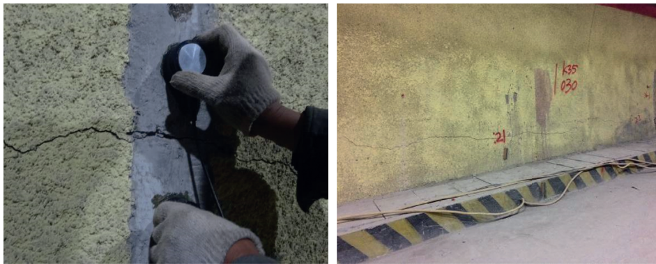
FIGURE 8: Longitudinal cracks of secondary tunnel lining.
