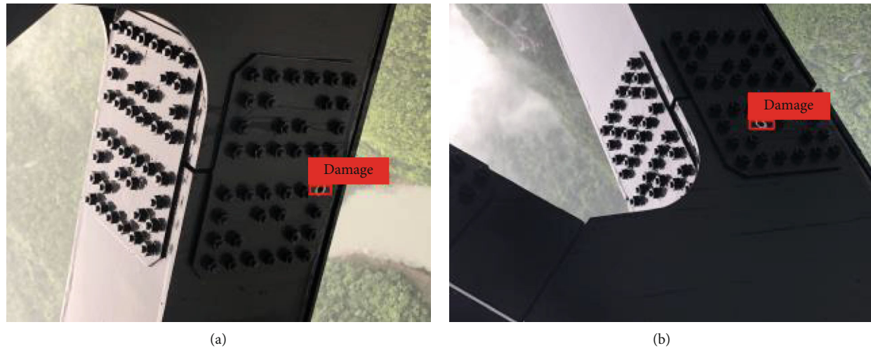
FIGURE 9: Detected bolt delayed fracture on an actual bridge.
