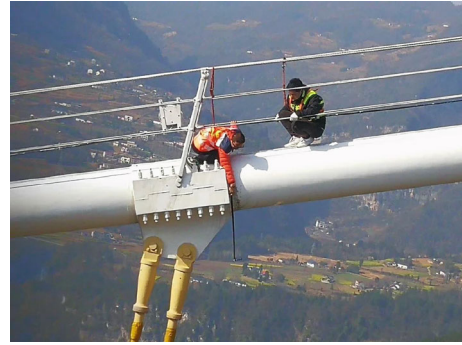
FIGURE 1: Maintenance workers are inspecting the bolt delayed fracture in a long-span steel bridge.
