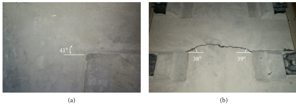
FIGURE 3: Distribution of cracks on the surface of track slab. (a) Initial crack. (b) Crack coalescence.
