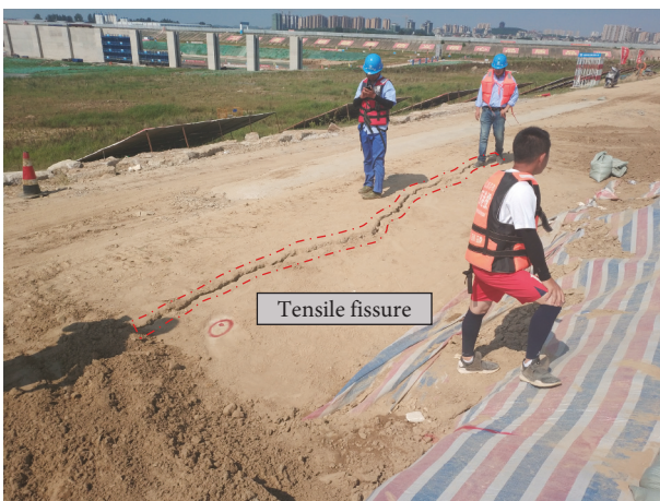
FIGURE 4: Tensile fissure at the top of upstream cofferdam.
