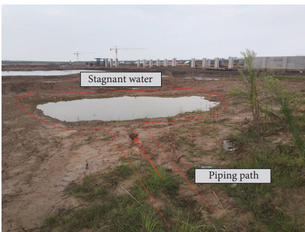
FIGURE 5: Piping effect at downstream face slope of cofferdam.
