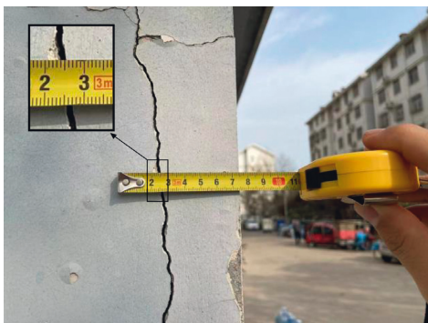
FIGURE 15: Cracks on the first floor of the masonry structure.
