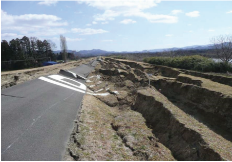
FIGURE 1: Damaged river embankment in the Edano area of Abukuma River [2].
