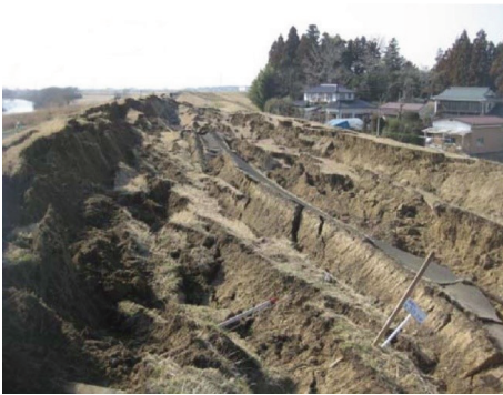
FIGURE 2: Damaged river embankment at Shimonakanome upper stream of Naruse River [2].
