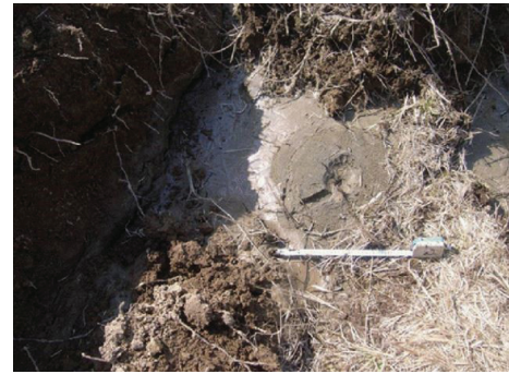
FIGURE 9: Sand boiling in the embankment crack [27].
