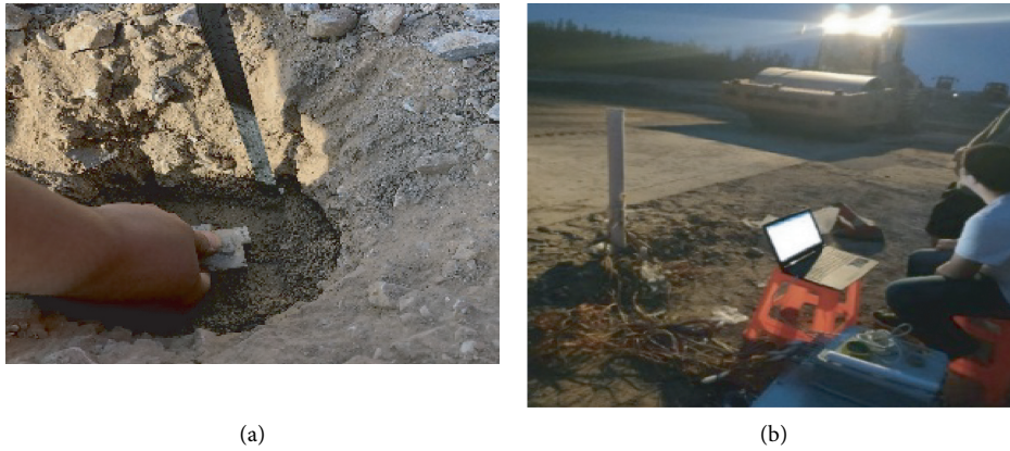
FIGURE 5: (a) Installation and embedment of sensors and (b) data acquisition in the field test.
