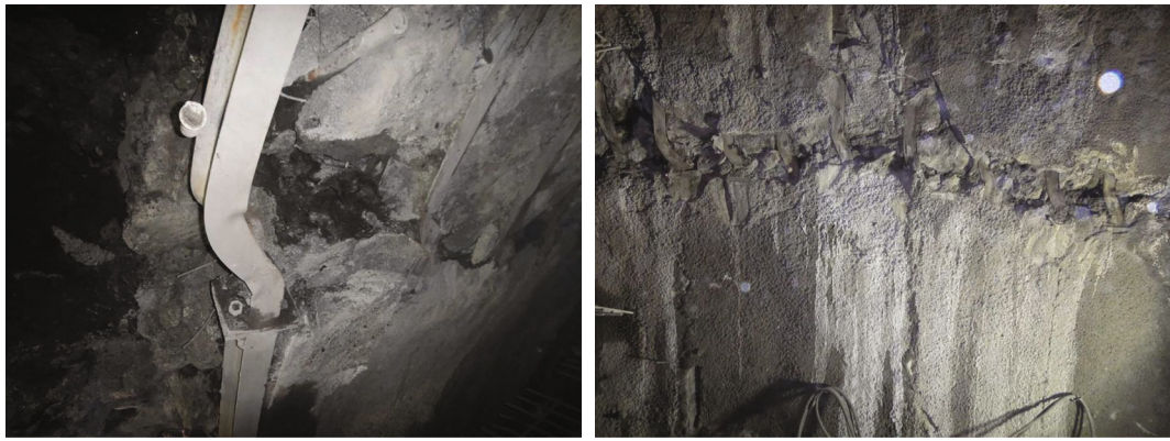
FIGURE 2: Distortion and spalling of shotcrete of steel frame for initial support of arch.
