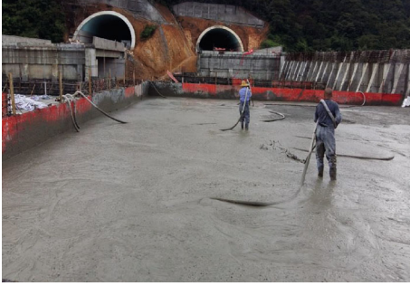
FIGURE 1: Use of lightweight foamed concrete as a filler behind buttressed earth-retaining wall.
