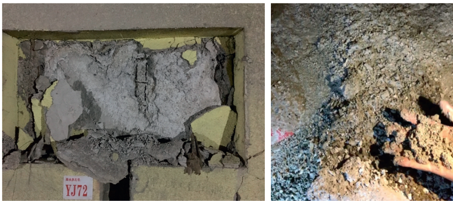
FIGURE 2: Photographs of the corroded tunnel lining concrete.
