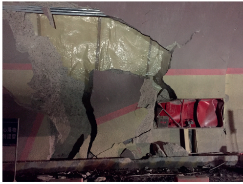
FIGURE 5: Sudden collapse of the secondary tunnel lining.
