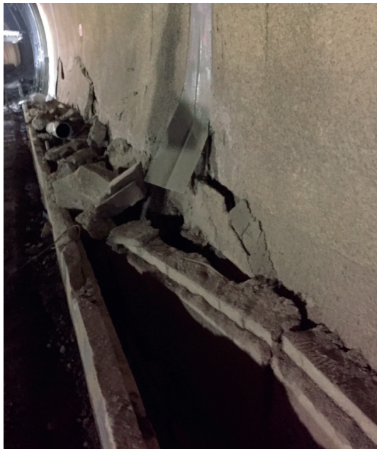
FIGURE 6: Inner wall extrusion of the cable trench.
