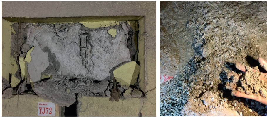
FIGURE 12: Photographs of the corroded tunnel lining concrete.
