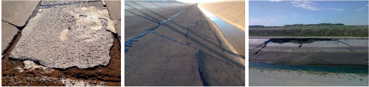
FIGURE 1: Typical damages of canals in northern China [2, 3].
