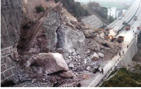
FIGURE 1: Collapsed highway slope.
