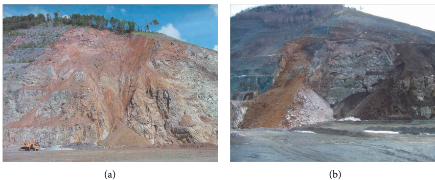
FIGURE 4: Slope failure that occurred at the quarry in (a) July 2004 and (b) April 2009.
