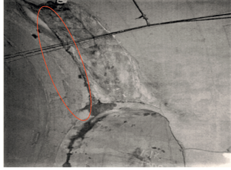
FIGURE 1: Lining crack of tunnel in chi-chi earthquake [4].
