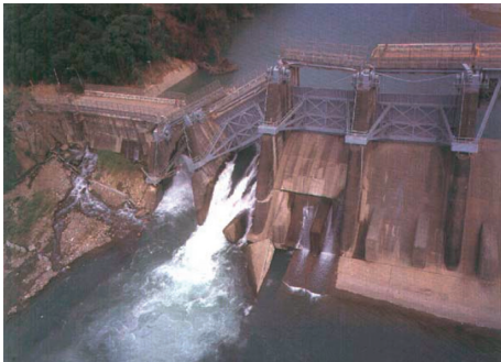
FIGURE 6: Dam damage caused by earthquake.
