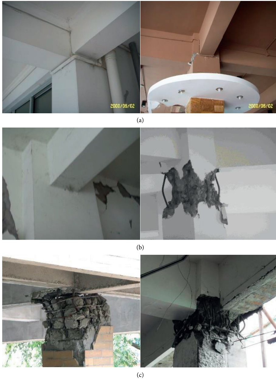
FIGURE 3: Damage to structural elements—beams and columns. (a) in good condition or slightly damaged. (b) Moderate damage. (c) Severe damage.
