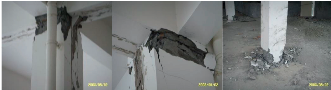
FIGURE 2: Damage to infill wall in the Lushan earthquake.
