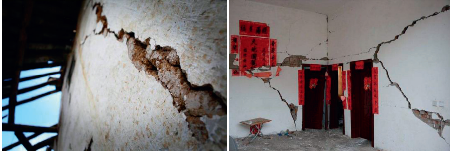
FIGURE 1: Damage to structural elements in the Wenchuan earthquake.
