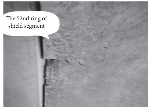
FIGURE 13: On-site segment damage.
