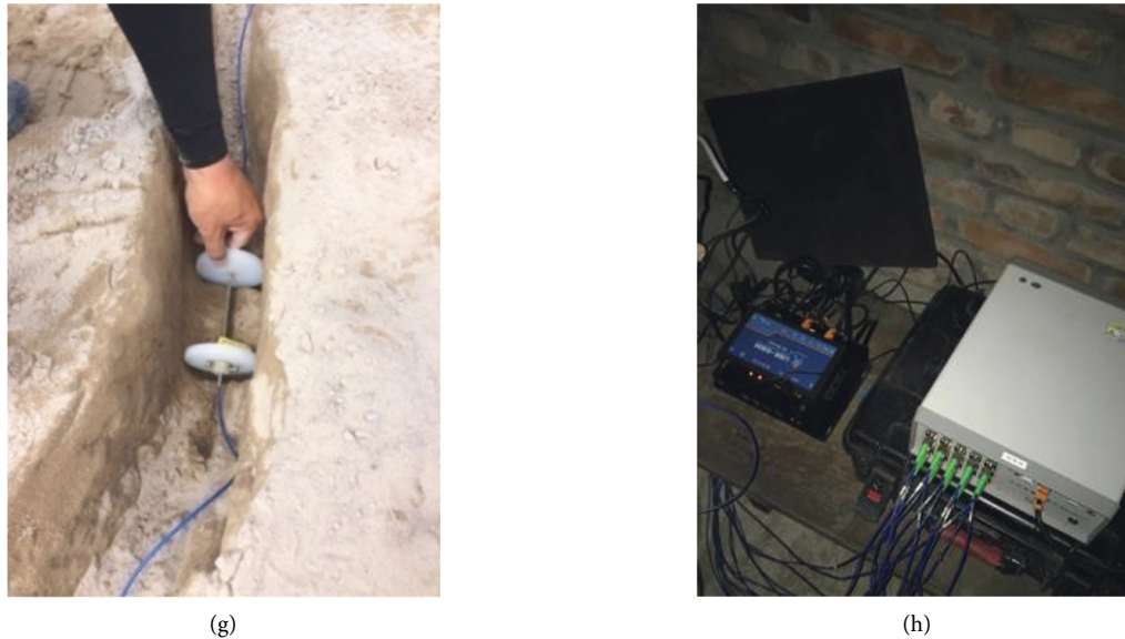
FIGURE 3: Temperature, humidity, and deformation sensors embedded in the test roadbed soil and data collection terminal. (a) Buried groove excavation, (b) fiber optic cable layout, (c) humidity sensor, (d) burying of humidity sensor, (e) humidity sensor data collection terminal, (f) fiber grating (temperature) strain sensor, (g) embedded fiber grating (temperature) strain sensor, and (h) strain sensor data acquisition terminal.
