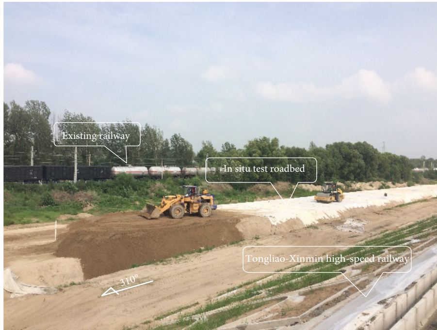
FIGURE 2: Spatial relationship diagram of the test roadbed and the railway under construction.
